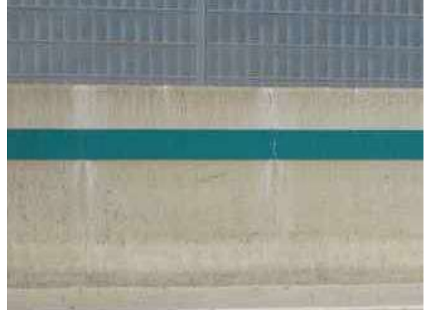
S3 방호벽 균열(0.2mm/1.5m)
