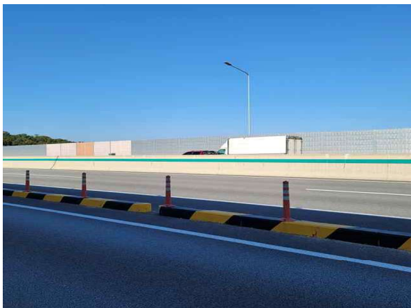
S5 균열 (0.2mm/1.5m×13EA)
