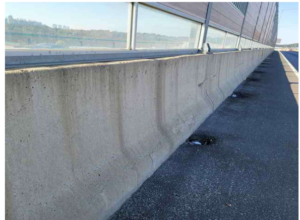
S5 균열 (0.2mm/1.5m×24EA)
