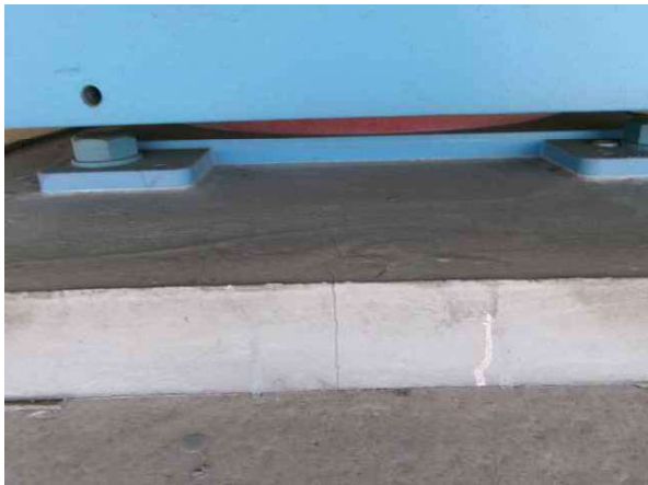
P2-Sh3 받침물탈 균열 (0.2mm/0.2m)
