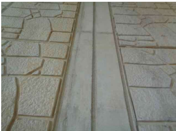
A2 균열 (0.2mm/5.5m)
