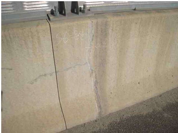
S6 균열 (0.2mm/1.5m)
