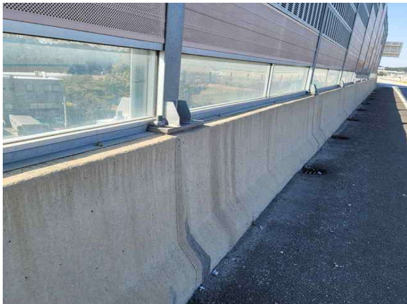
S7 균열 (0.2mm/1.5m×6EA)
