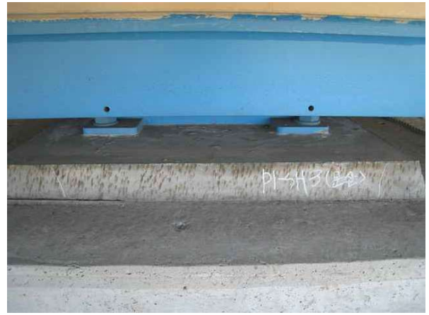
P1-Sh3 받침물탈 균열 (0.1mm/0.1m×3EA)
