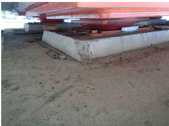
P5-Sh7 받침물탈 파손 (0.1m×0.1m)
