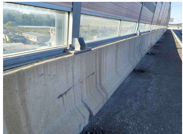
S6 균열 (0.2mm/1.5m×12EA)
