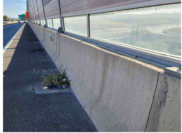
S3 균열 (0.2mm/1.5m×16EA)
