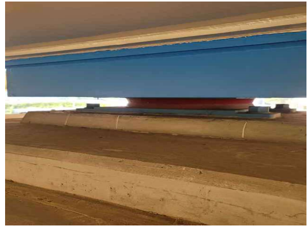
P1-Sh2 받침물탈 균열 (0.2mm/0.4m×3EA)
