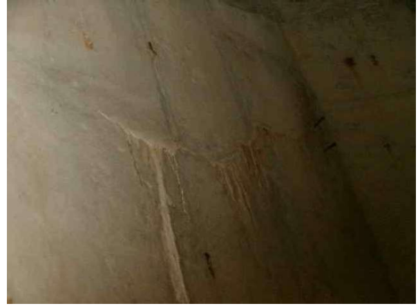
A1 균열부백태 (0.2m x 1.5m)
