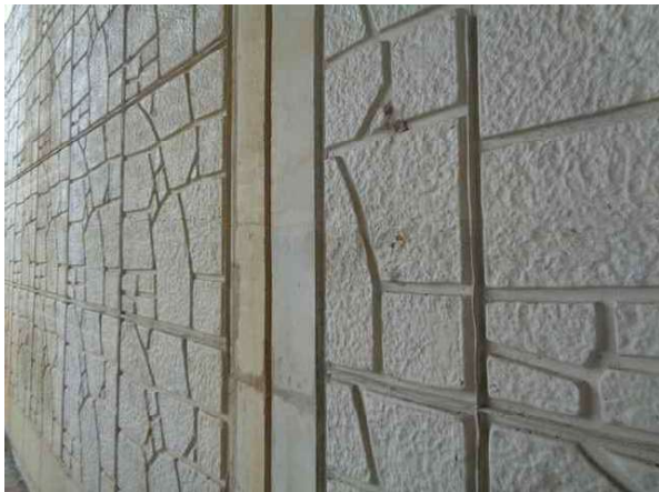
A2 균열 (0.2mm/3.0m)
