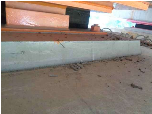
P2-Sh10 무수축물탈 균열 (0.1mm/0.2m)
