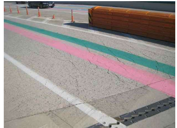
S2 접속도로 망상균열(5.5m × 4.0m)
